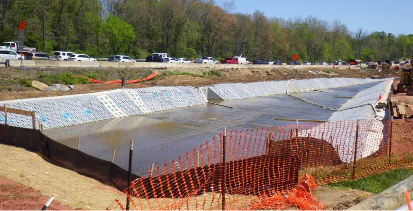
Fig. 4. A recently constructed massive drainage channel replacing a section of 1960s-relocated Colvin Run in Fairfax County, Virginia. Leesburg Pike (Rt. 7), shown in photo center, is being doubly widened. A large Piedmont / Northern Coastal Plain Basic Seepage Swamp (USNVC: CEGLo06406) runs along the south side of the above channel outside of the right photo frame. Despite the denuded, degraded landscape, the concrete channel is the only way to confine and accommodate enormous quantities of stormwater runoff from the widened roadway and environs without transferring it to forested wetlands and stream valleys, especially with 72" culvert outfalls aimed at said wetlands (middle left of photo). Photo by R.H. Simmons.
